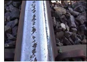
Severe Rail Center Spalling
