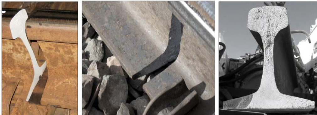
Broken Base – Transverse Photo Examples of Broken Base - Transverse
